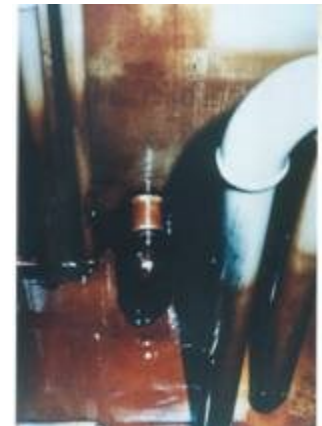
Dirty maintenance environment
