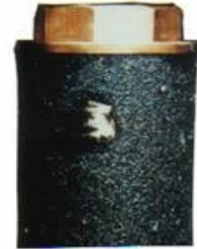
Filter or strainer blockage
